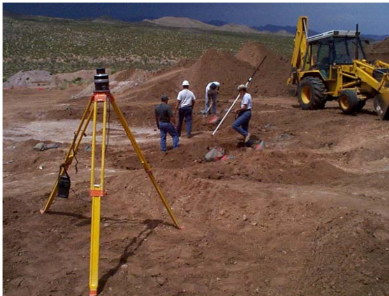
Figure 5-1. Photograph of the excavation of the testbed, showing the use of shovels to help determine the extent of the highly damaged region. The photograph also shows the 3-D surveying systems used throughout the tests.
